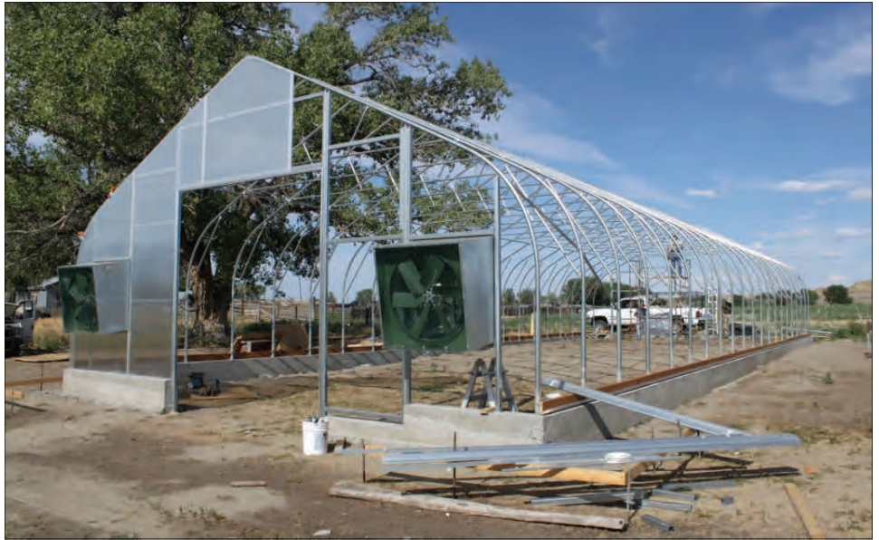
A high-production garden grow tunnel under construction at Pine Hills Youth Correctional Facility in Miles City
