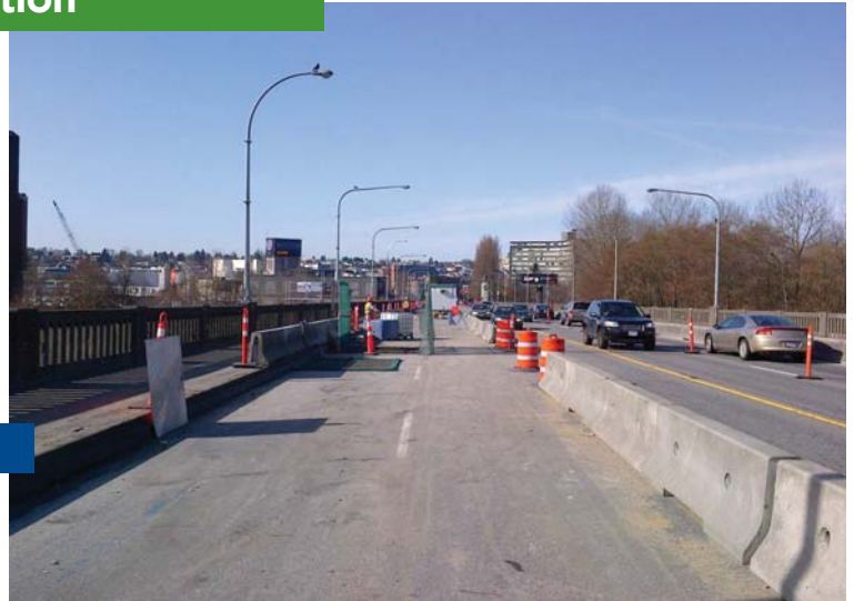
During construction, travel impacts may be similar to when the previous round of Burrard Bridge repairs were made in 2014. Typically, three motor vehicle lanes, two bike lanes, and one sidewalk were kept open.
